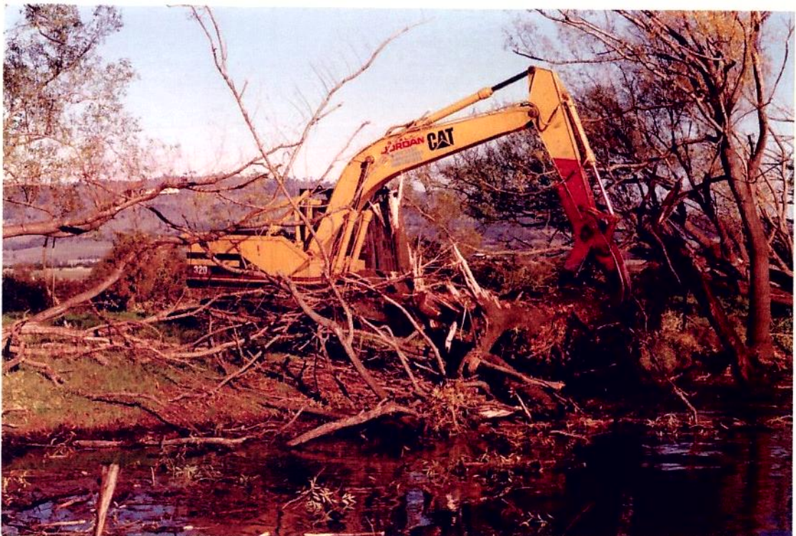
Willow clearance with excavator with crab grab (Woodland Management, G. Jordan, Liffey). Large log being removed for stacking, Eliza Farm, Campania, April 1999.
