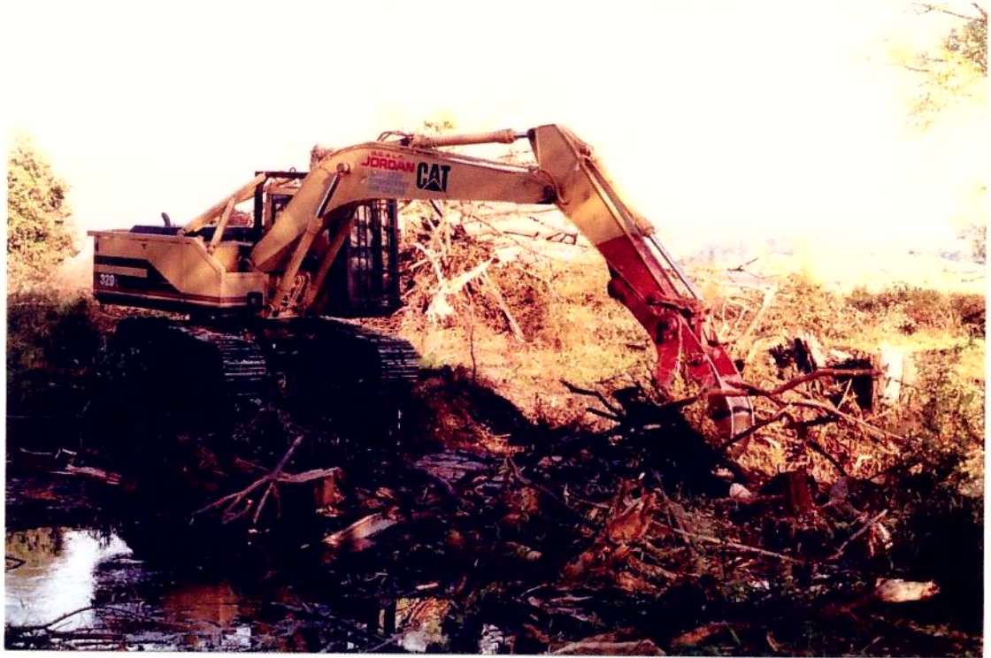
Excavator removing branches and debris from Coal River, Eliza Farm, Campania. Stumps in the river will be removed, those on the bank painted with herbicide and left for stabilisation.
