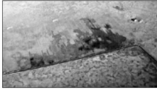
Leaking channels have been identified as an important source of water loss from a conveyance or distribution system.
